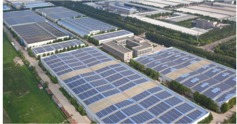
Commercial & industrial distributed PV station
