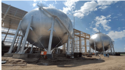
Compressed air energy storage
